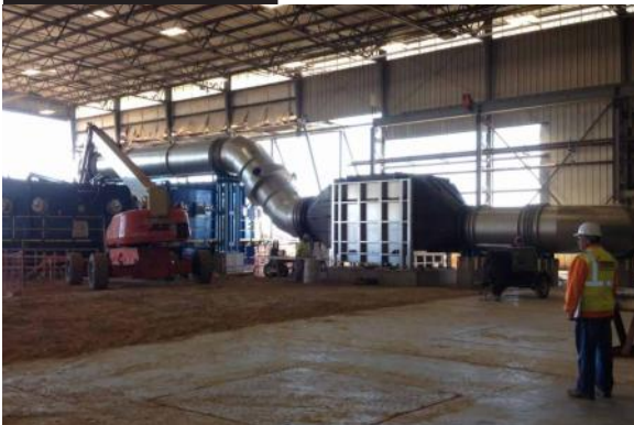
Photo above shows the rotary hearth furnace and the rotary hearth furnace stack and recuperator at the PTC Seamless Pipe Mill in Hopkinsville, Kentucky.
