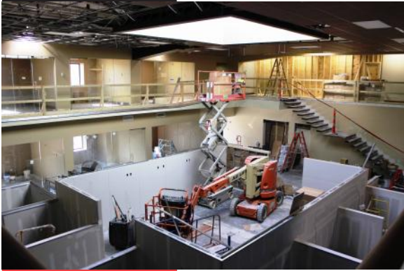
Photo above shows the new construction department office suite, which is currently being constructed at the Robinson Construction headquarters in Perryville, MO.
