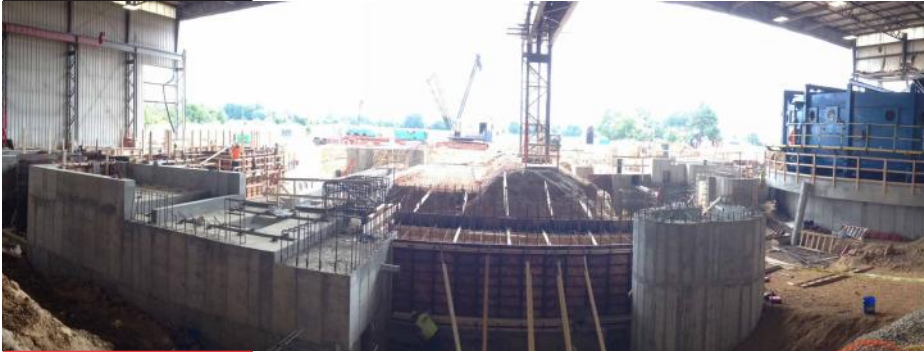
Photo above shows work in progress by Robinson Construction on the rotary hearth furnace, piercer foundations, scale water trench foundations (formed), and pilger foundations at the PTC Seamless Pipe Mill in Hopkinsville, Kentucky.
