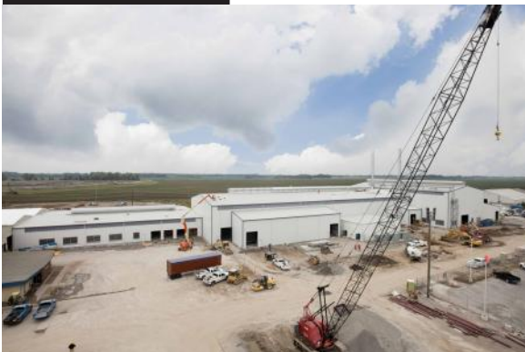
Photo above shows the Rod Mill 3 Buildings project at Noranda Aluminum in New Madrid, MO. The project included construction of 7 pre-engineered metal buildings totaling 88,000 sq ft.
